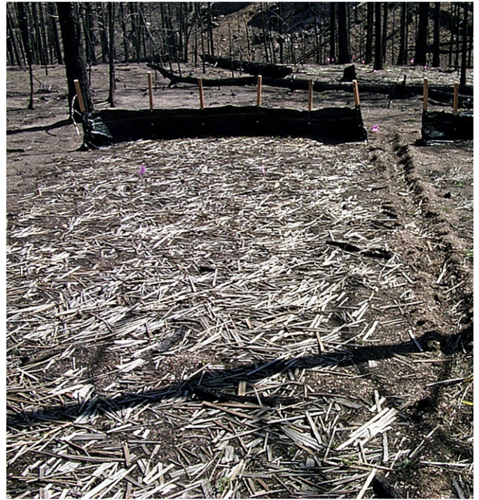
Fig. 2. A wood strand mulch plot at the Hayman fire. The photo was taken immediately after plot installation from the top of the plot looking downslope into the fence.
